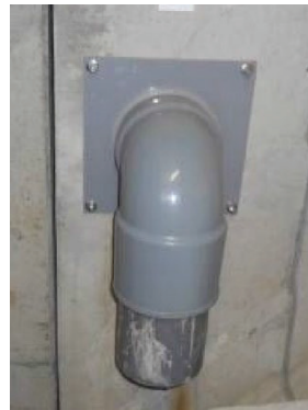
Figure 2: Joint drainage hole (example of shape that enables measurement at each hole)
