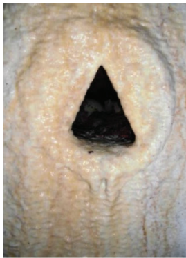
Figure 1: Free lime adhesion to joint drainage hole
