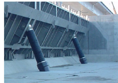
Steel Flap Gate with Hydraulic Cylinders
