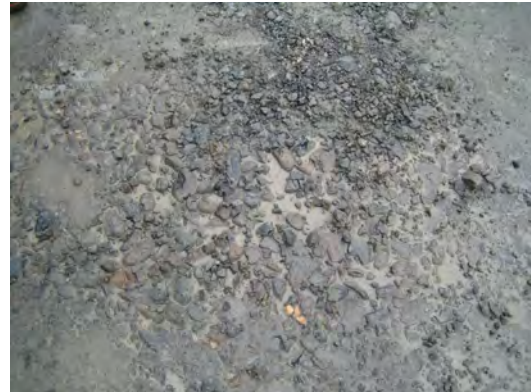
Fig.7 Segregation of large size aggregate, because of deterioration of workability under the hot weather
