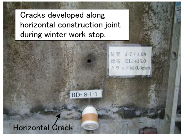
Fig.-6 Micro cracks at the upper surface
