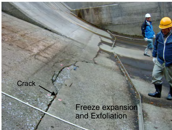
Fig.-5 penetrated cracks at the dam toe
